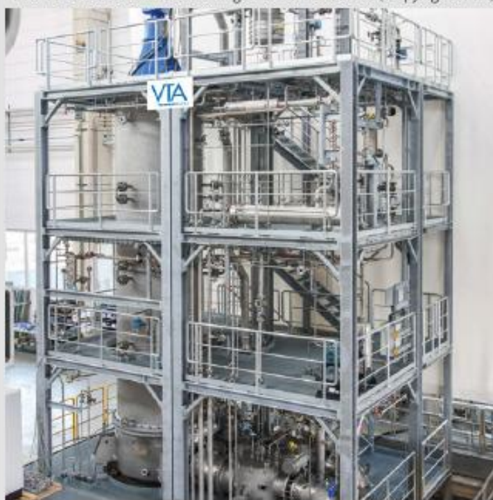
Figure 1: Industrial SPD plant supplied to Nutriswiss AG by VTA Verfahrenstechnische Anlagen GmbH & Co. KG (Copyright: VTA)
